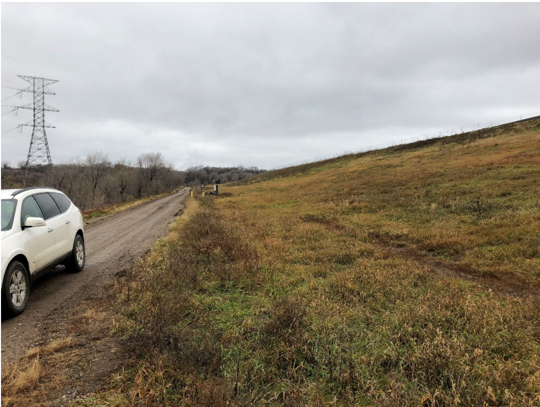
Photo 26: Location 11 – Looking Northwest, Cell 2C & 2B Southwestern Waste Slope and Anchor Trench
